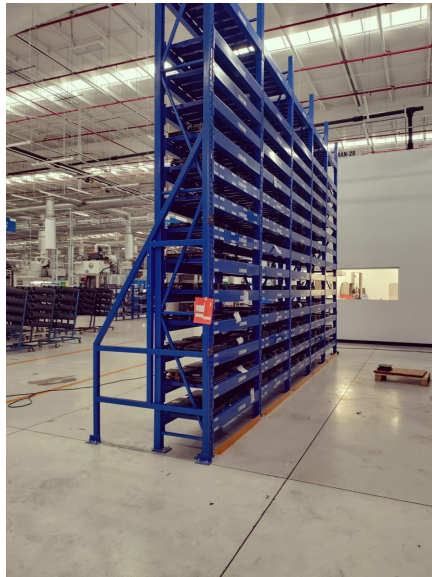
Rack industrial multinivel instalado en planta automotriz · Multi-level industrial rack at automotive plant
